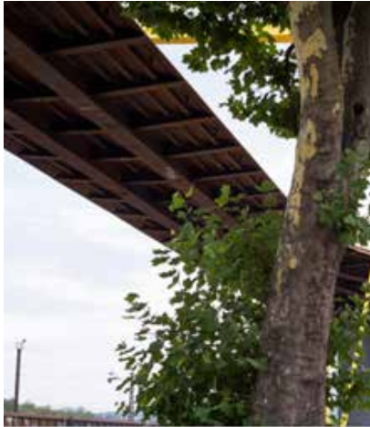
View of the bridge from below, showing its steel structure and the curves in the route.
